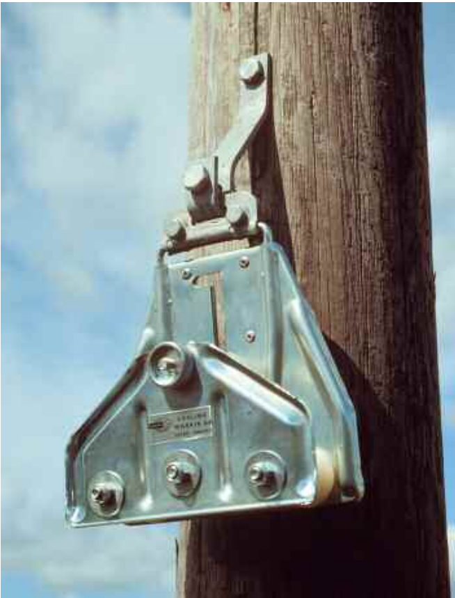
Line rollers for fibre optic.
